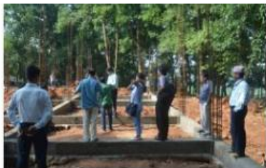
Supervision and Monitoring by Consultant Engineer and Donor Representative at OPD Building Construction site of Rapti Eye Hospital
